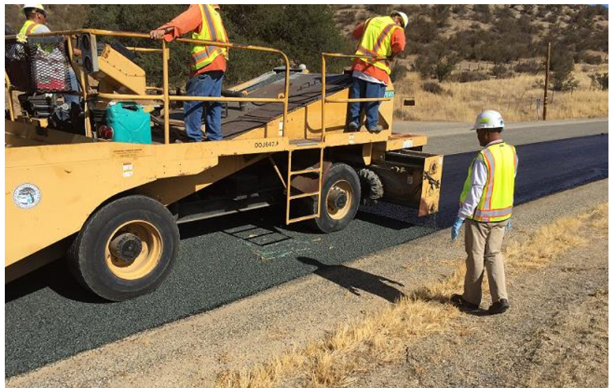
RMA Public Works crews at work on one of its many chip seal projects. Chip sealing is the process of pavement treatment that provides a new road surface and seals minor cracks.
