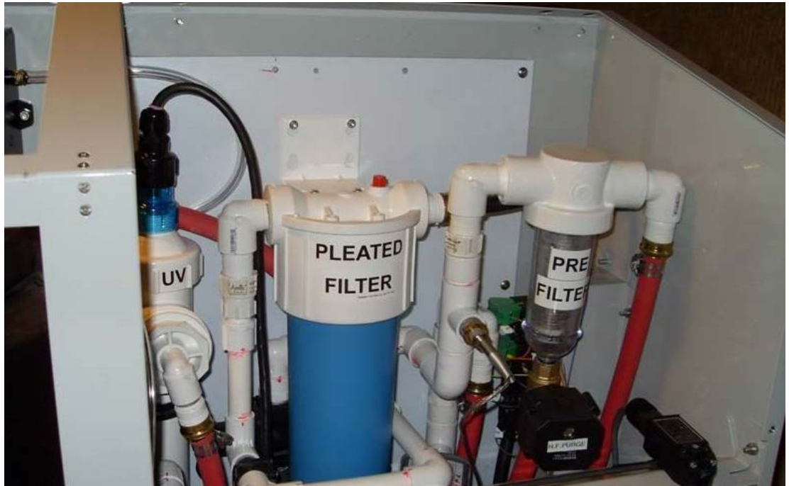
Disinfection, filtration and pre-filtration components (l-r above) of the indoor gray water reuse system given first-ever approval by Environmental Health staff.
