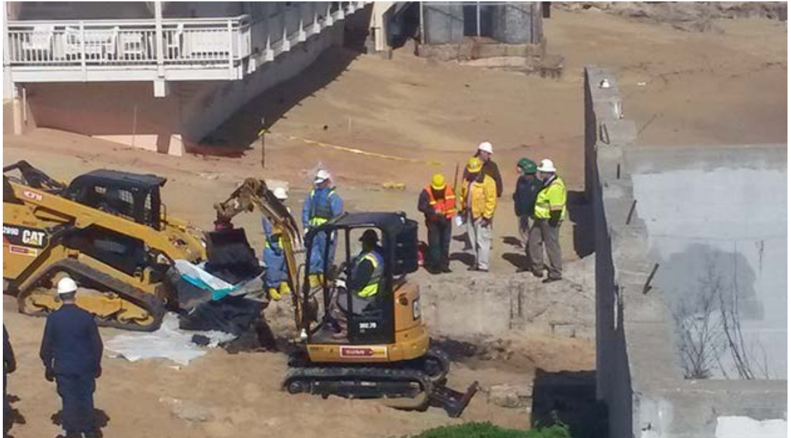
Work crews excavate the area near a mysterious oil leak near Cannery Row last month.
